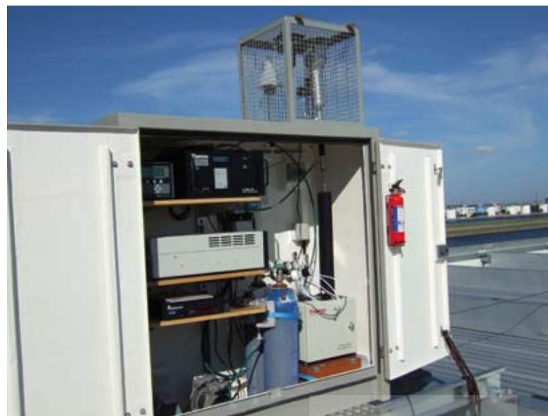
Air Quality Monitoring Equipment at London City Airport
