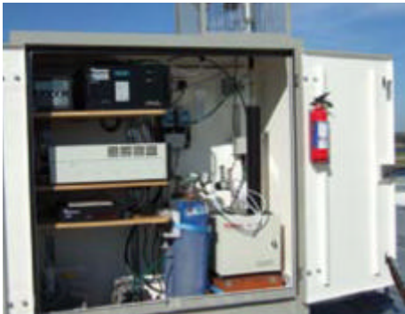
Air Quality Monitoring Equipment at London City Airport
